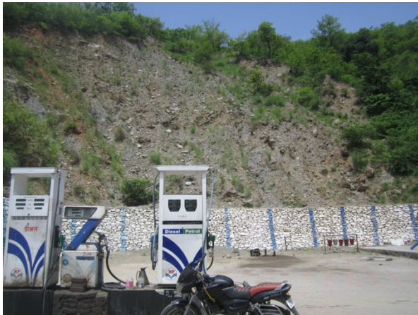
Plate9. Lingui 3 landslide caused loss to petrol pump
