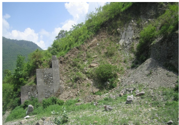
Plate12. Buinth 2 landslide-reactivated old landslide
