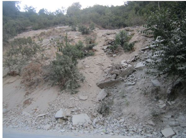
Plate10. Saur landslide due to road section cutting
